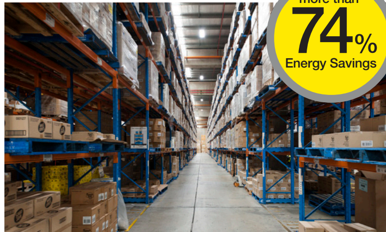
Aglo Europa Linear LED Flatbay installed in storage aisle
